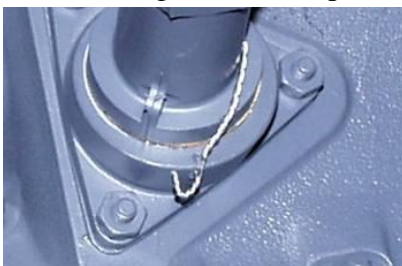
Figure 2 Safety Wire on the Oil Level Gage
