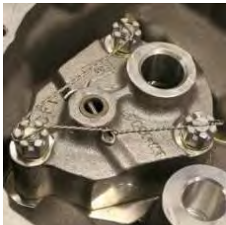
Figure 3 Safety Wire on the Oil Pump
