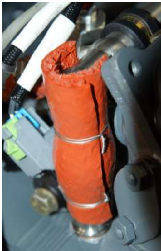
Figure 11 Installed Fire Sleeve P/N 01M29869
