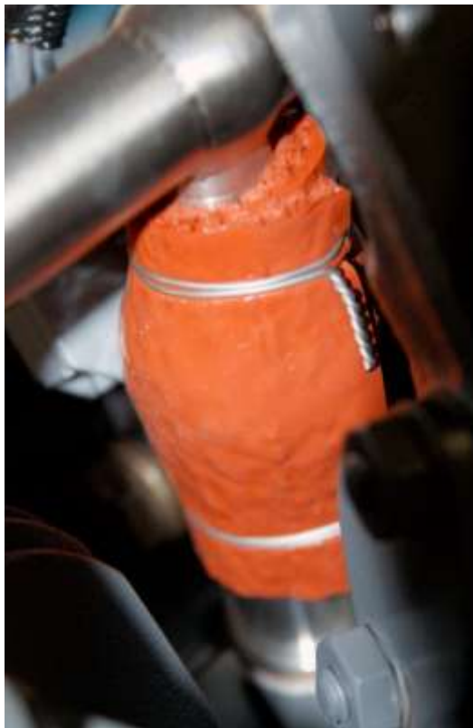
Figure 10 Installed Fire Sleeve P/N 01M29868
