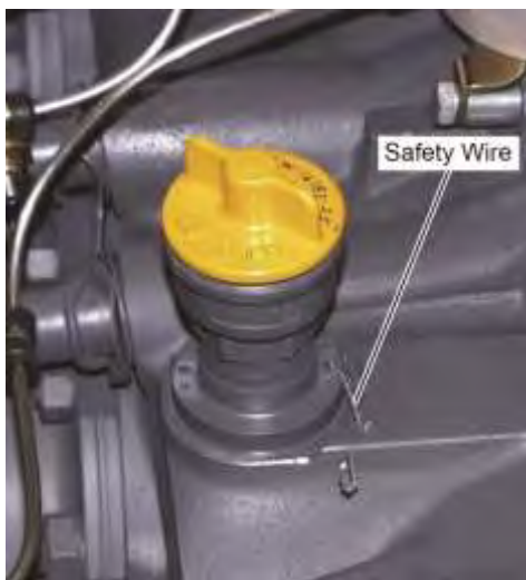
Figure 2 Safety Wire on the Oil Filler Extension
