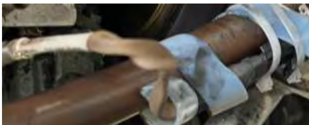
Figure 37 Incorrect Installation Cable is Twisted
